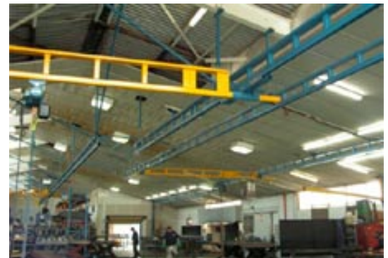
Multiple cranes at an industrial equipment manufacturer. Several of these cranes were relocated from a previous site.
